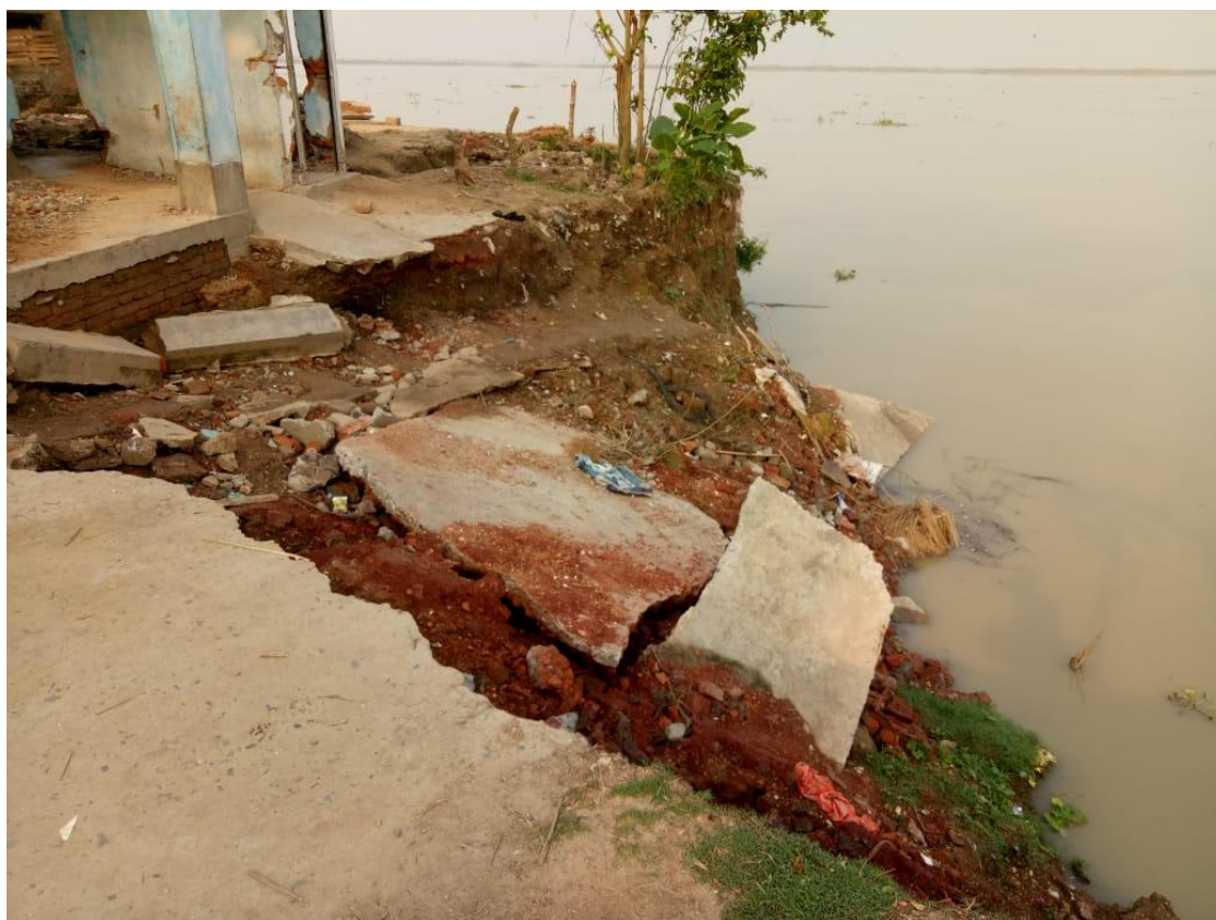
Image No 101 : Collapsing of Pucca Houses, School Building Because of River Action, Birnagar G.P
