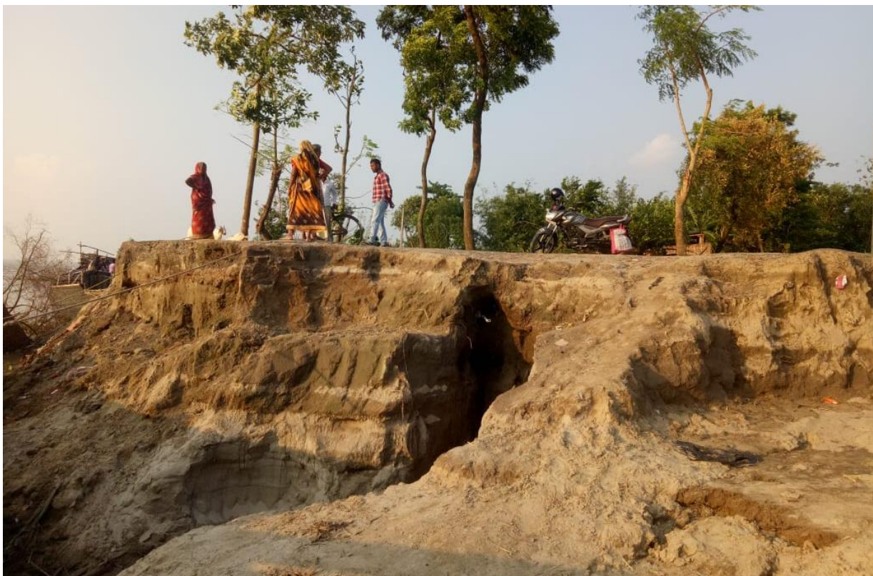
Image No 98 : About 150 Houses were Washed Off Because of Heavy October Rainfall at Birnagar Sarkarpara 24°50'21.24"N 87°57'5.46"E
