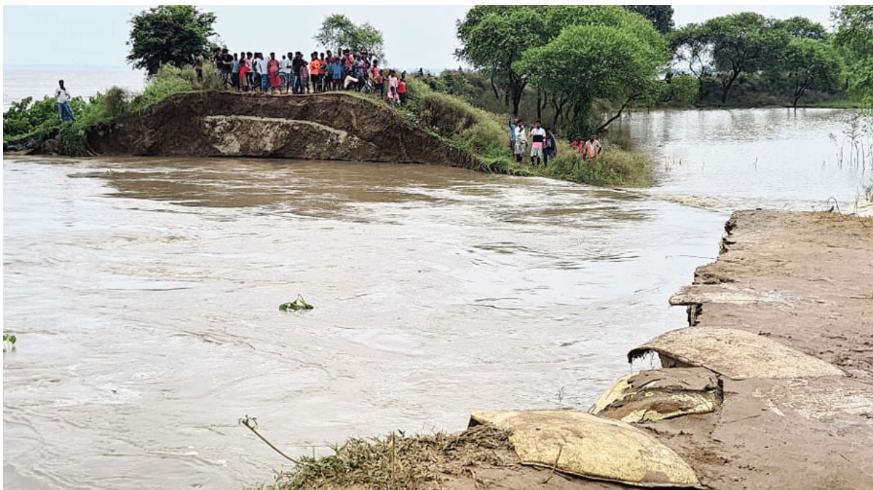
Image No 36 : Breaching of Embankment at Bhutnir Char, Source : The Telegraph 2020
