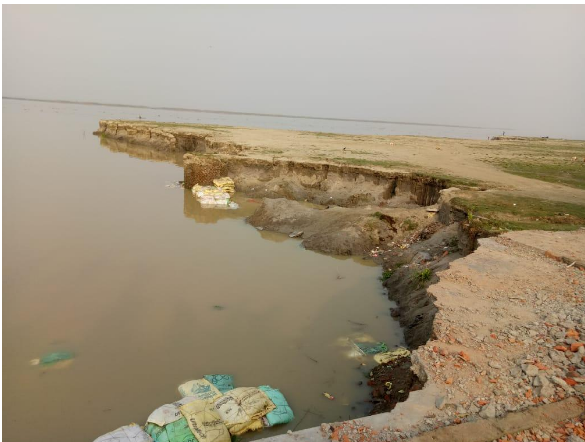
Image No 103 : The Eroded Bank of Ganges, Kaliachak
