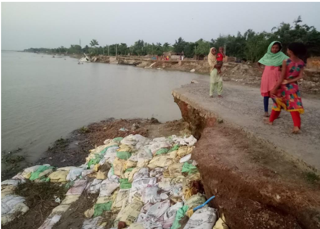
Image No 40 : Heavily Eroded bank of Birnanagar II G.P area, 24°50'55.96"N 87°57'30.85"E
