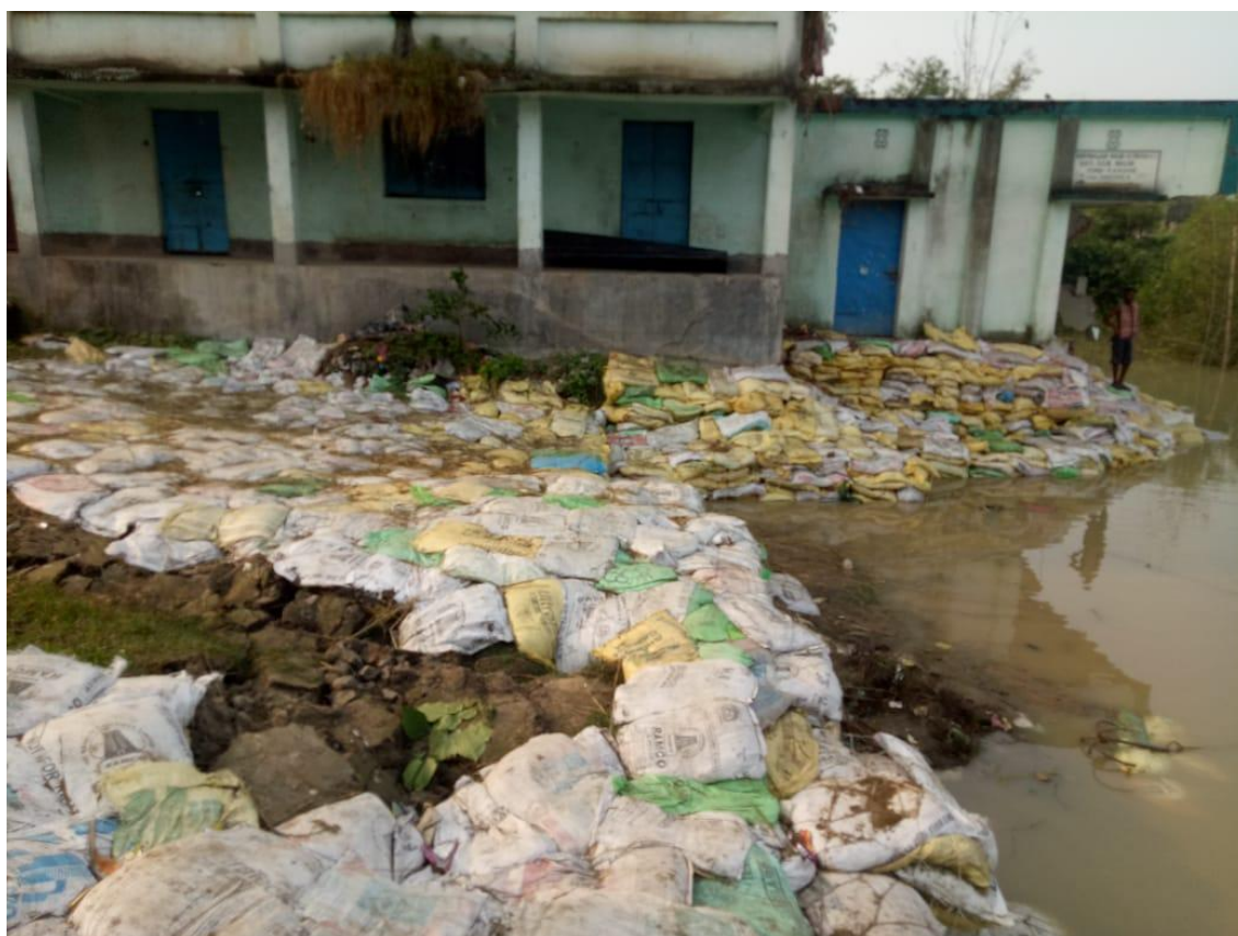
Image No 102 : Collapsing of Pucca Houses, School Building Because of River Action, Birnagar
