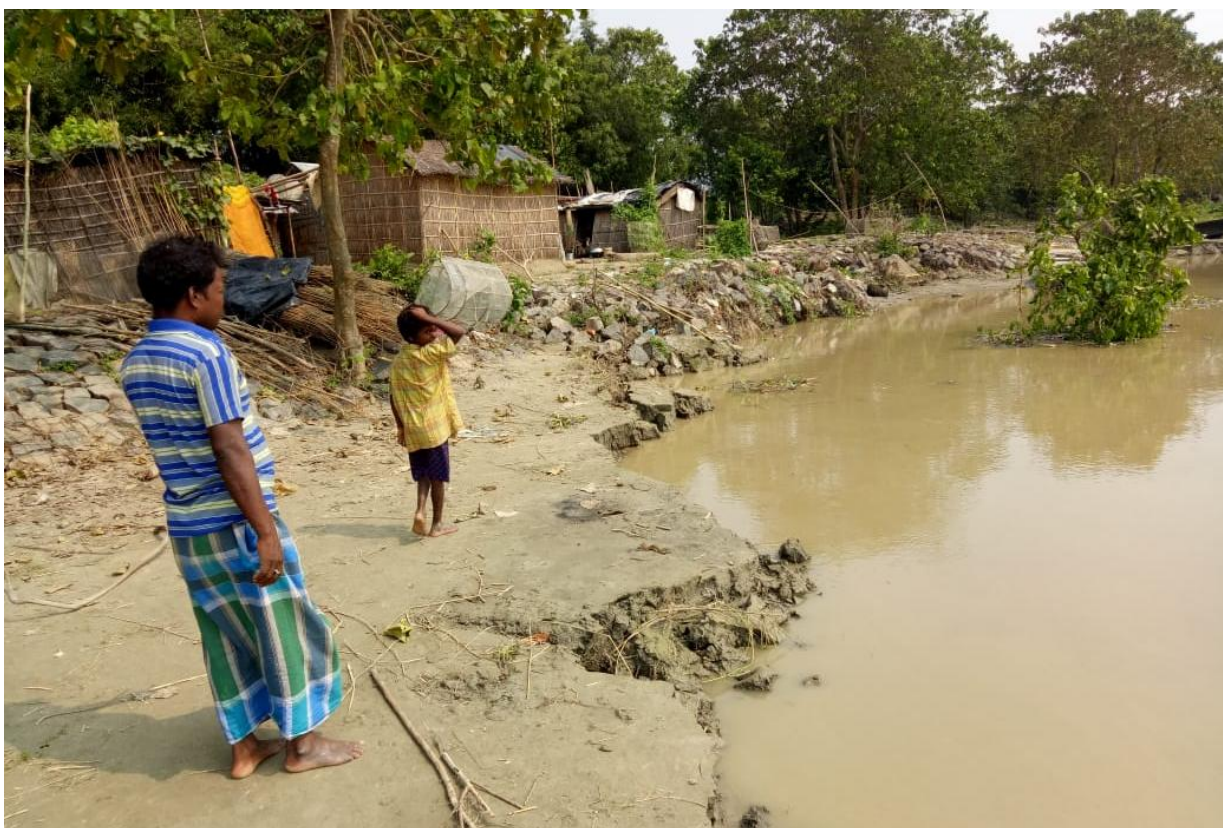
Image No 27 : Heavily Eroded Bank of Narayanpur Village Near Manikchak Ferry Ghat
