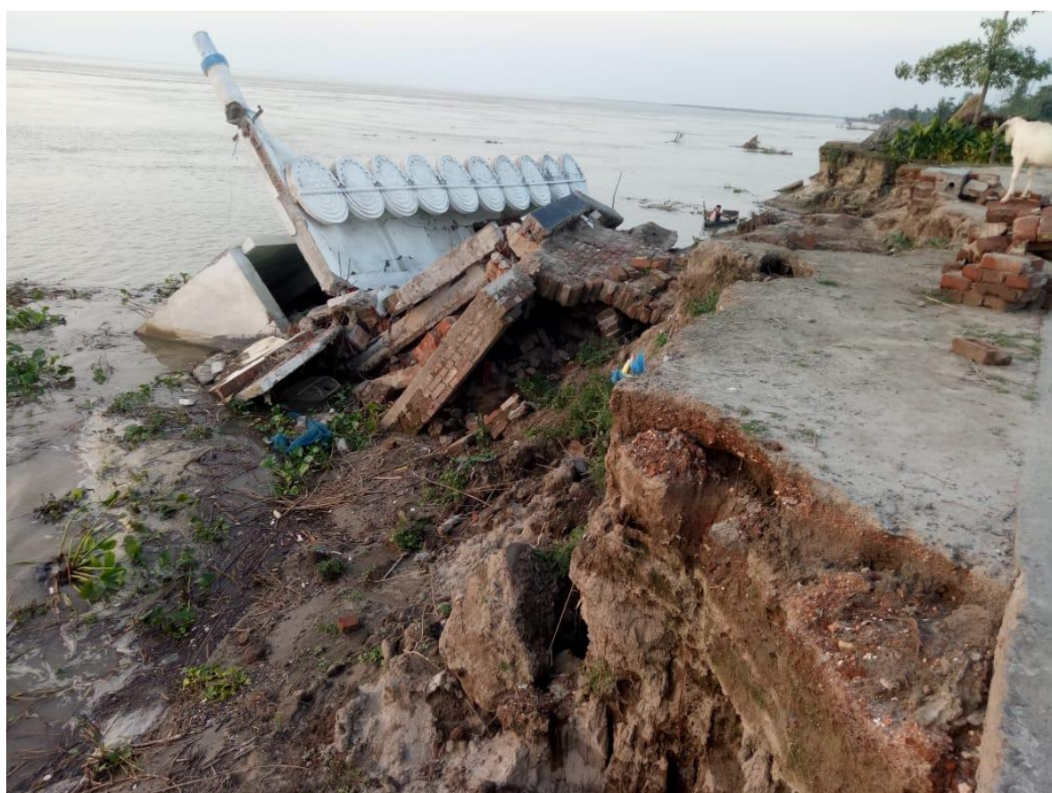
Image No 105 : Bank Erosion and Damaged Structure at Saheb Nagar - Kanchantola
