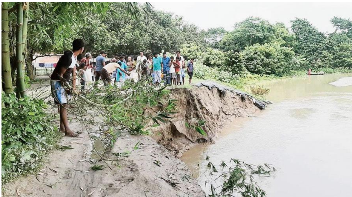
Image No 104 : An Instinct for Self-preservation has Prompted Residents of Saheb Nagar-Kanchantola, a village in Manikchak block of Malda district on the banks of Kalindri river, to team up and prevent erosion caused by the river, without waiting for measures by the state irrigation department.
