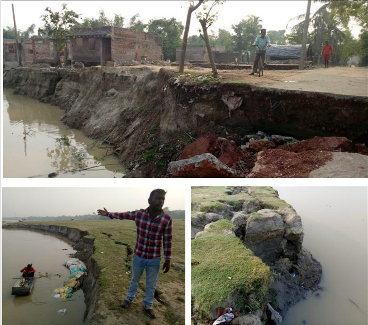
Image No 33 : Bank Erosion at Sarkaritola, Birnagar I Gram Panchayet
